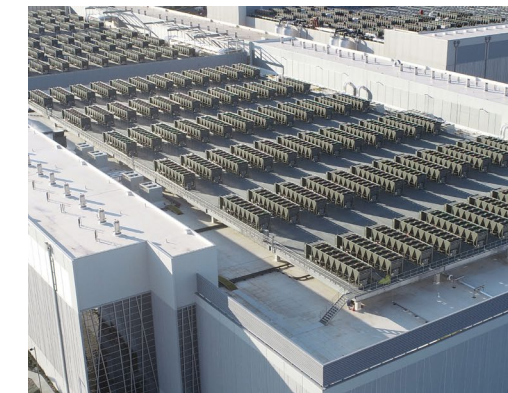
LC1 Data Center Data Center in Loudoun County, VA. Craftsmanship Award & Washington Building Congress
